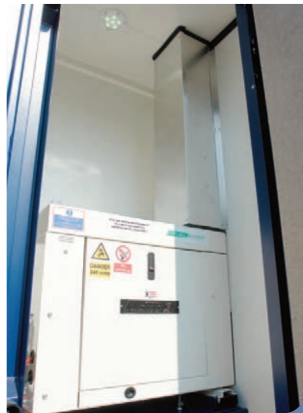
Easily accessible Generator
