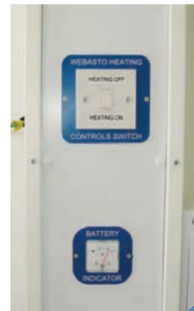
Heating On/Off switch and Battery Indicator
