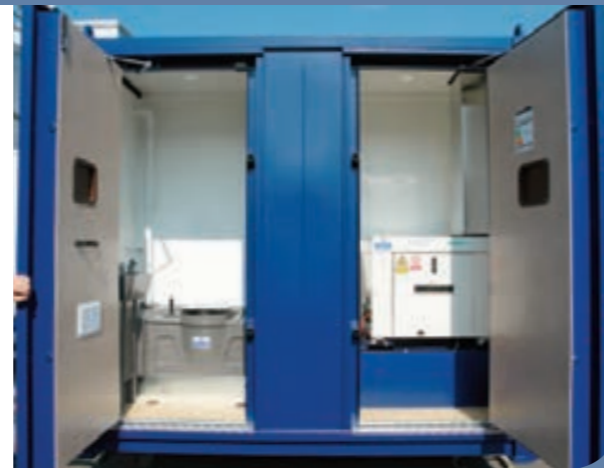
Generator & Toilet Area
