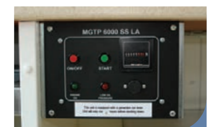
Generator Start/Stop control panel
